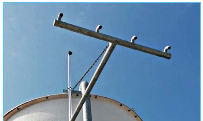
2 Scarico a bandiera in ferro zincato Galvanized pipe system with nozzles for discharge
